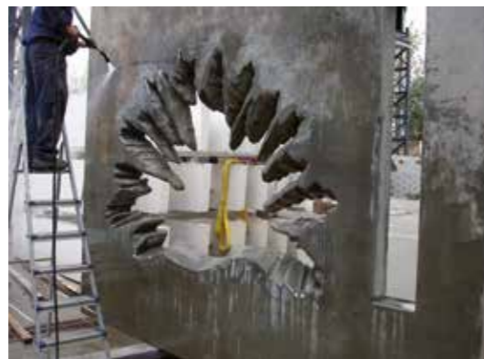
Hotel Renaissance, Hospitalet de Llobregat. Molde del panel armado de la fachada interna / Reinforced panel mould for interior facade.
